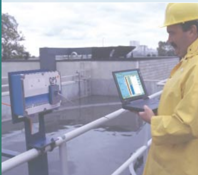
By installing the DPS 300 with Dolphin Plus, an operator can "see" the sludge level profile to verify unit performance.
